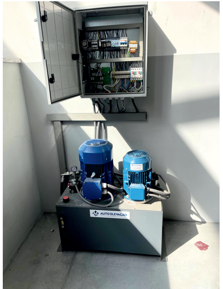
Central Hidráulica e Quadro Elétrico Hydraulic Station and Electrical Panel
